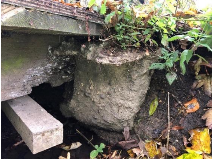
Eroded VB footpath bank, concrete and wood foundation
